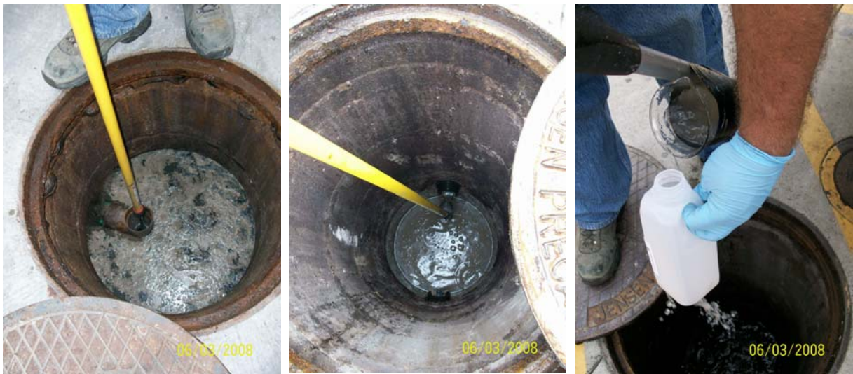
Samples collected from grease interceptor effluent tees and sample boxes
